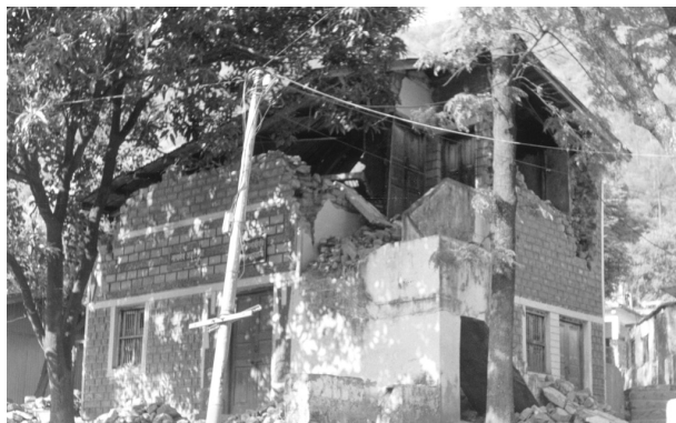
Figure 7.1 : A Damaged Building Due to an Earthquake
